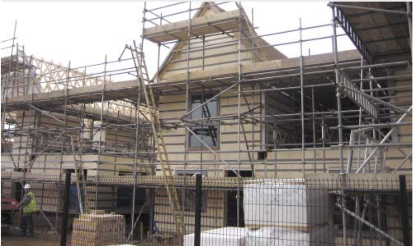
Homes using the polarwall insulated concrete formwork system are being constructed alongside those using traditional block construction, which enables accurate comparison of construction process and lifetime performance.
